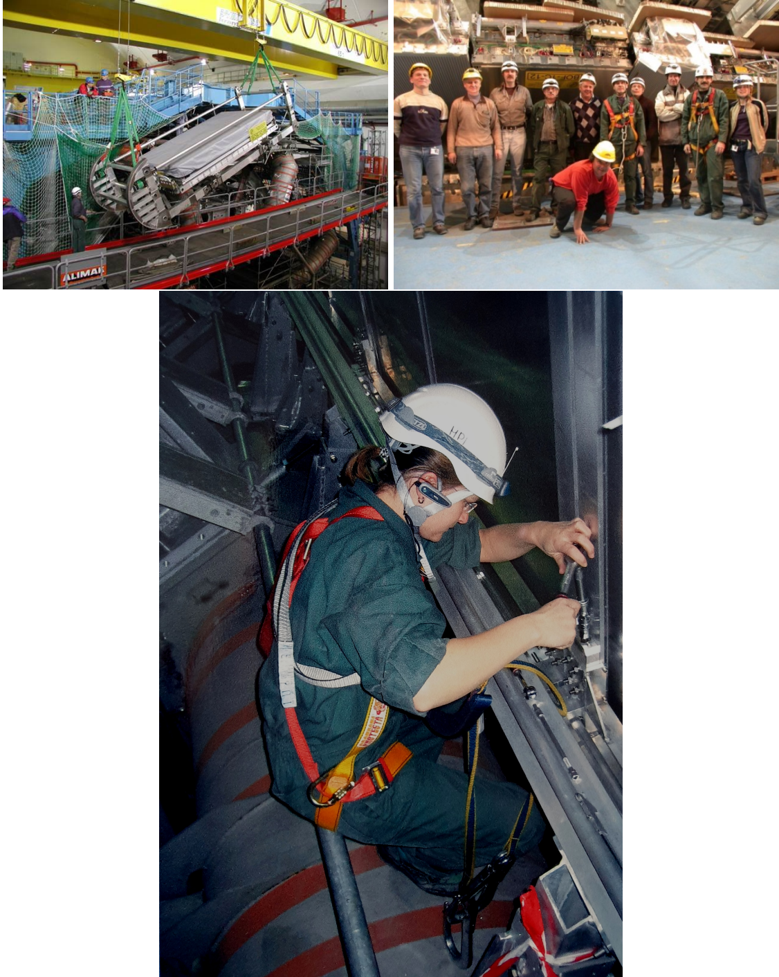
Figure 31: Top Left: Installation of an MDT chamber on the outside of a barrel toroid magnet cryostat at the top of the ATLAS detector. The chambers had to be lowered to the ATLAS cavern, inserted on rails mounted on the toroid coils and positioned with millimeter precision. Top right: Installation team of the MPP MDT chambers in the "feet" region of the barrel muon spectrometer on the floor of the ATLAS experimental cavern. Bottom: Fine adjustment of an MDT chamber in the ATLAS muon spectrometer by a young female technician from MPP working in climbing harness at large height and in very cramped space.
